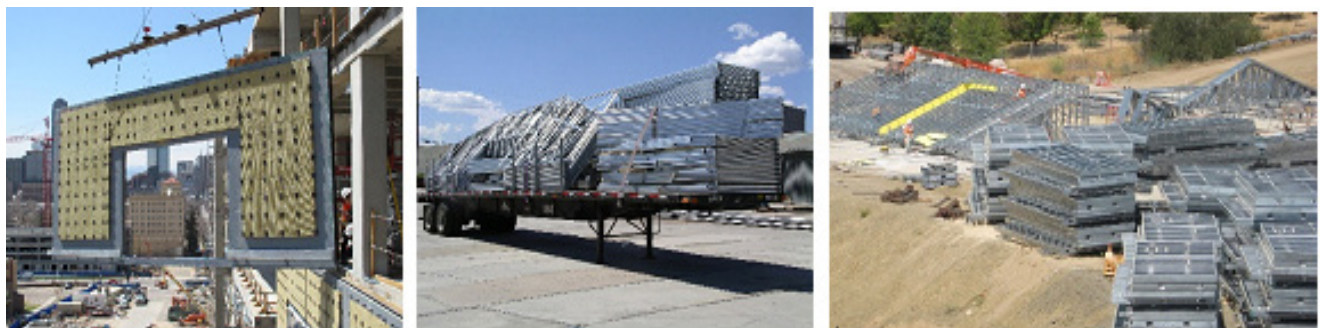
CFS panel construction (Left to right: exterior wall panel installation, CFS panels ready for shipping, Panels on construction site waiting installation).
